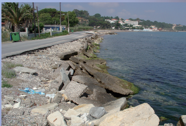
Coastal erosion in the area of intervention (Patraic Gulf, Western Greece)
